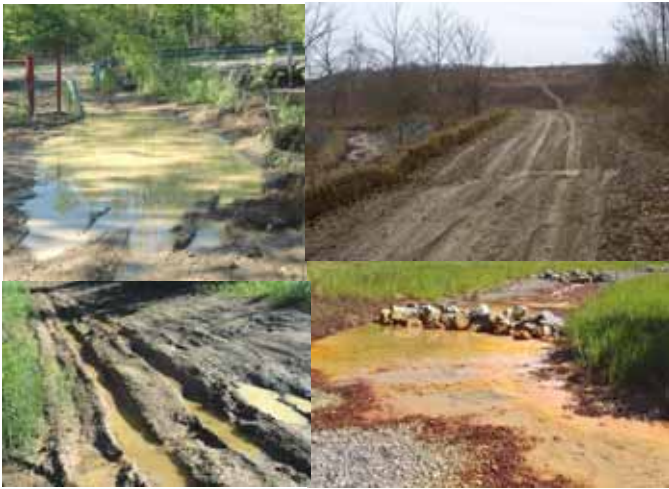
Vandalism & Erosion Impact At Site
